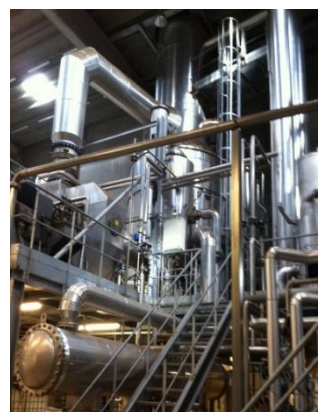
Photo 1. Falling film evaporator (France Evaporation ©)
