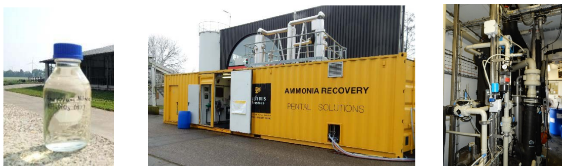
Figure 7 Ammonium nitrate solution (left) from the stripping-scrubbing installation (middle & right) during the WINGS project.
